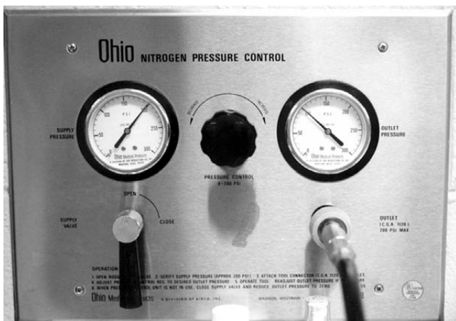
Figure 89-2 OR wall outlet for nitrogen gas.
